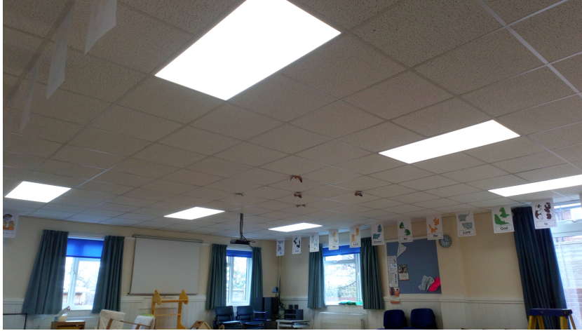
Fig 7: LED lights installed at Pinhoe Road Baptist Church
